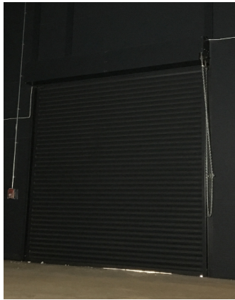
roller shutter door interior
