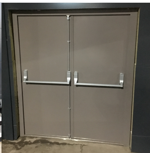
fire exit doors interior
